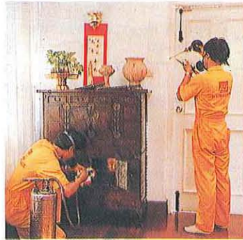
Termite control in the house
