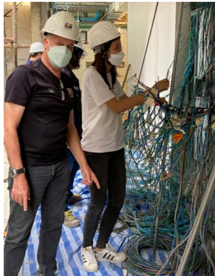
▲ Chris and Pann check the wiring
